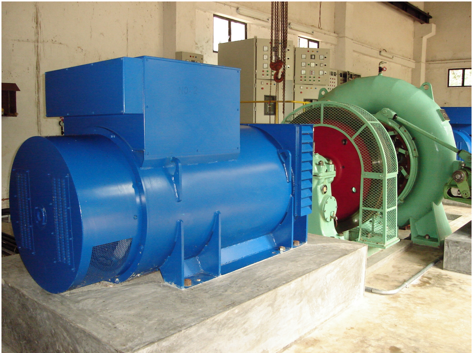
Fig. 19.1. Small hydro power plant (one unit 1250 kVA).
