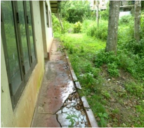
Figure 1 -damage to pavement due to tree roots.
