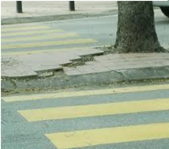
Figure 3 -damage to road due to tree roots.
