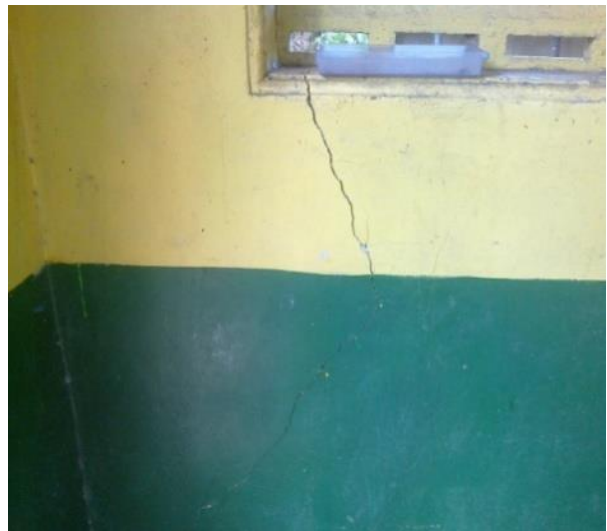
Figure 4 -damage to wall due to tree roots.
