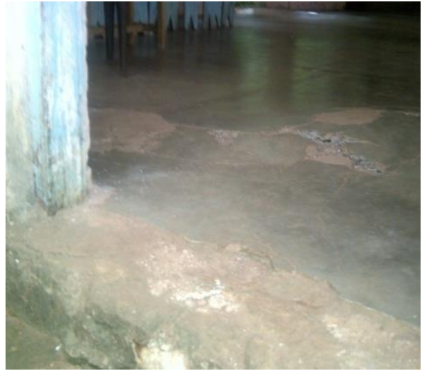
Figure 2 -damage to floor due to tree roots.
