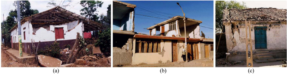
Figure 1. Out-of-plane failure: (a and b) collapse of masonry walls, and (c) failure of a wall connection (Mayorca 2001).
