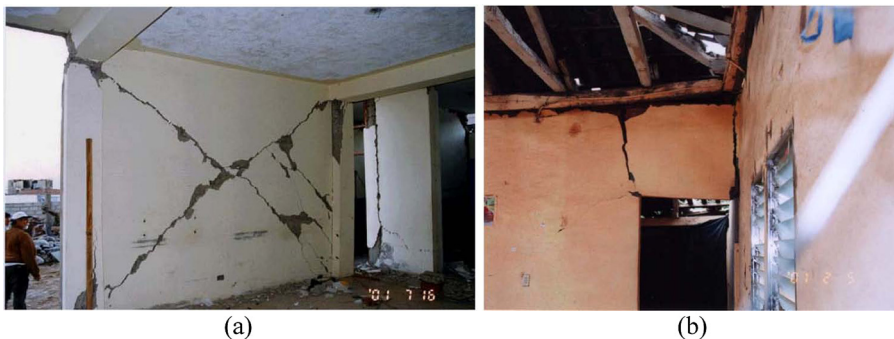
Figure 2. In-plane cracking of unreinforced masonry walls (Meguro et al. 2001).
